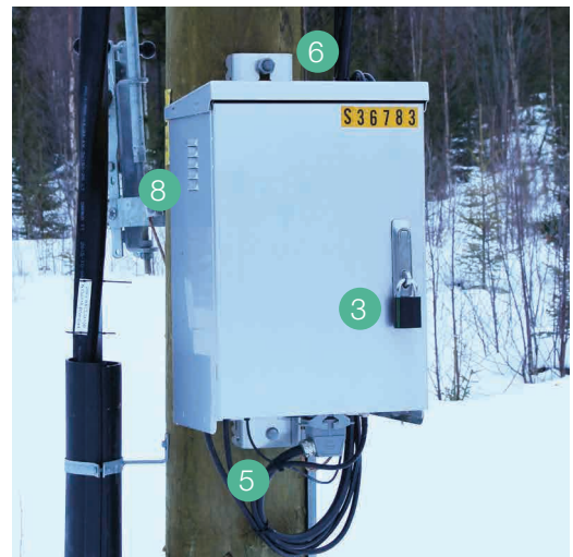
FTU recloser control cabinet
